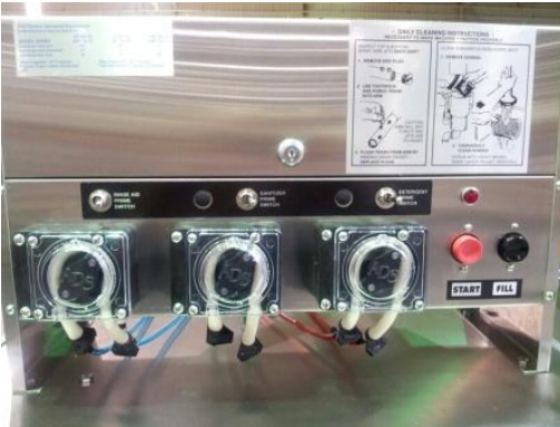
Showing chemical detergent, rinse, sanitizer external pumps
