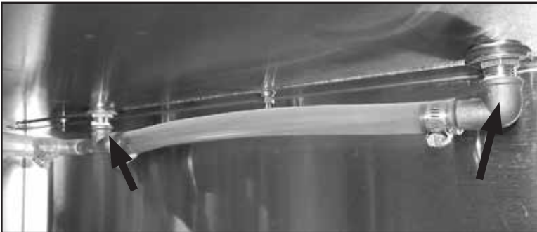
Fig. 20 - Connect flushing nozzle piping.
