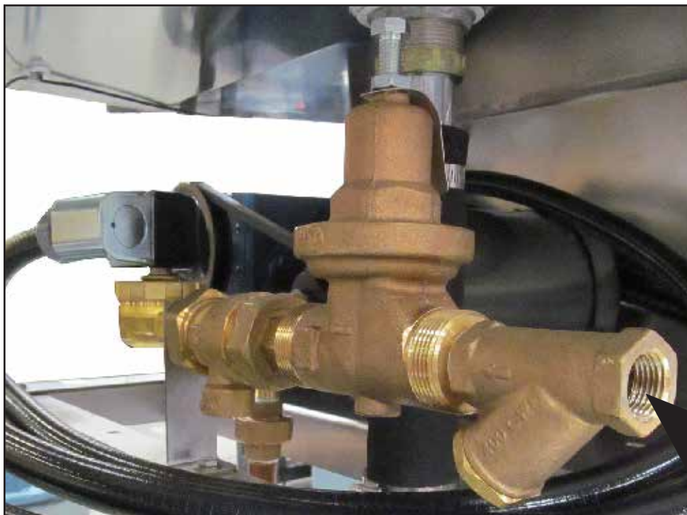
Fig. 21 - DWT 1/2" NPT cold water connection.
