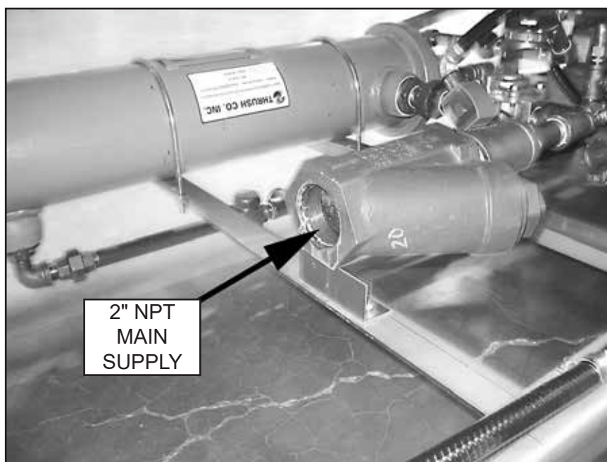
Fig. 27 - Main Steam Supply Line is 2" NPT
