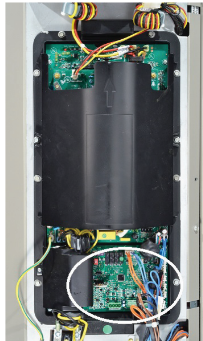
Figure 27 – Panneau de commande AOC (Application Operational Control)
