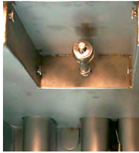
Upper float switch.
