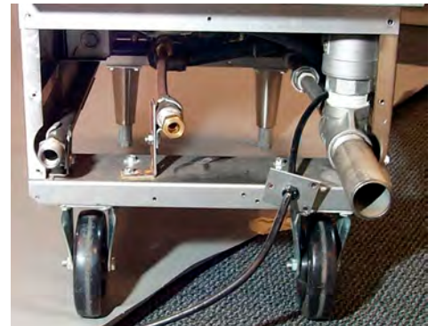
Gas fitting (from left), water hookup and drain.
