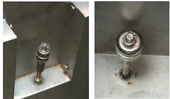
Figure 1: The float switches (above and right) should be cleaned periodically to eliminate starch buildup, which can impede the motion of the floats. Care must be taken, however, to ensure the shafts are not dislocated or the movement of the float hindered.
