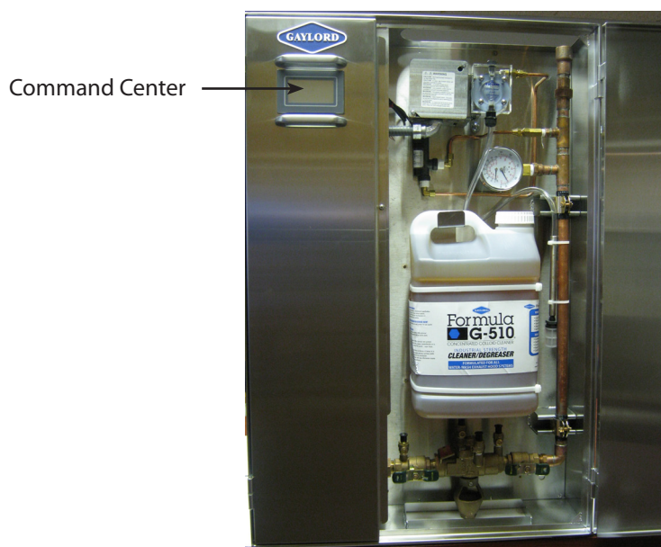
Figure 2-15-1 Wash Control Cabinet
