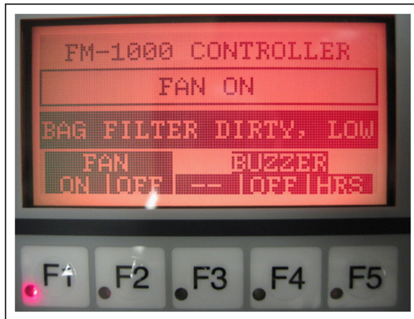
FIGURE 18-1 DISPLAY PANEL DIRTY BAG FILTER CONDITION
