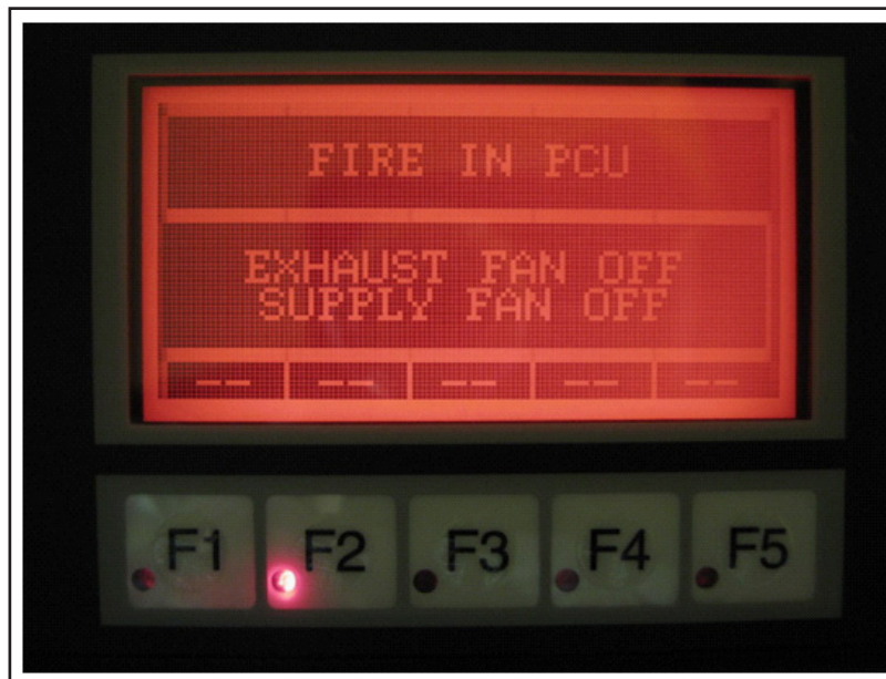
FIGURE 21-1 DISPLAY PANEL FIRE IN THE PCU CONDITION
