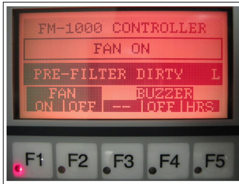
FIGURE 17-1 DISPLAY PANEL DIRTY PRE-FILTER CONDITION
