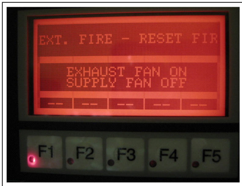
FIGURE 23-1 DISPLAY PANEL EXTERNAL FIRE CONDITION RESET SYSTEM
