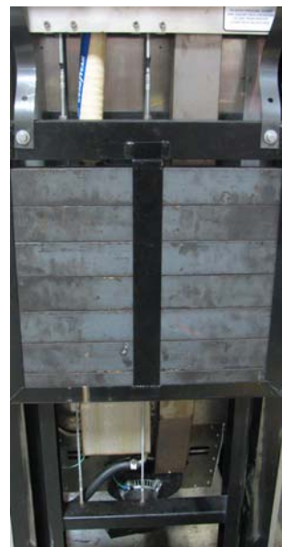
View of the counter-weights with cover removed
