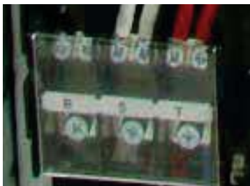
Measure Input Voltage.
