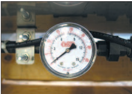
Gas Pressure Gauge P/N 16036 (On side of broiler)
