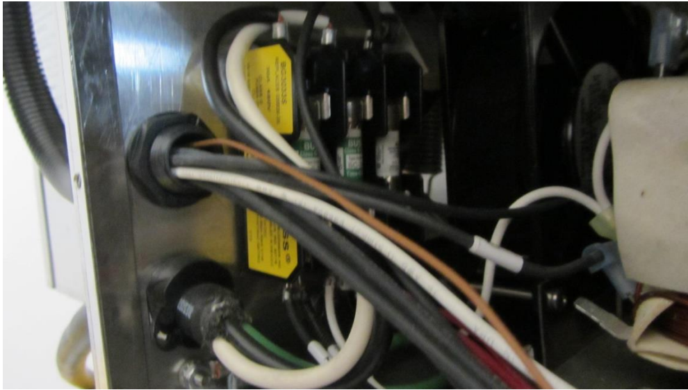
LINE FUSES (30A) – INTERLOCK FUSE (20A)
