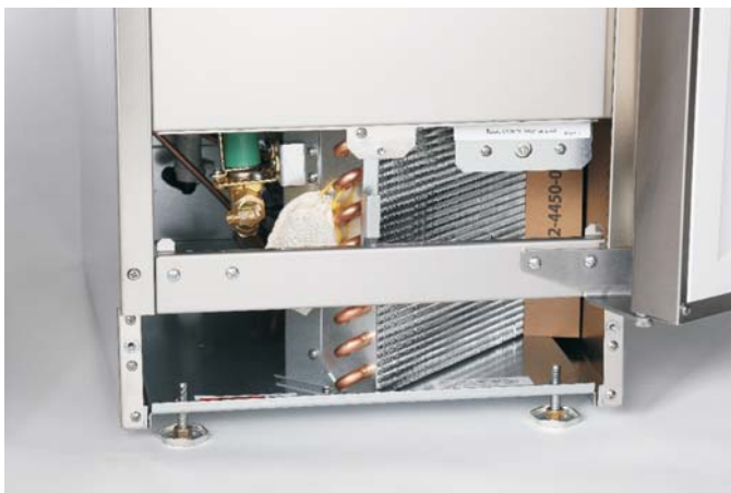
Inlet Water Solenoid Valve
