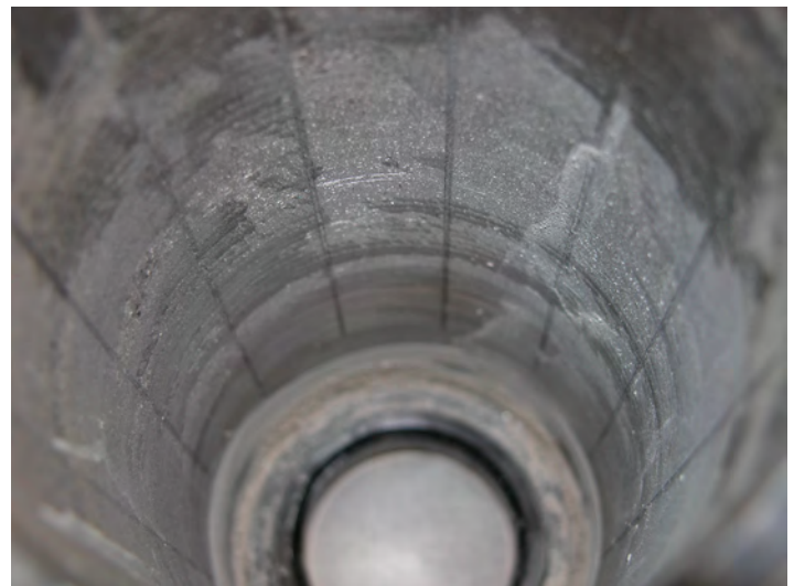
Example of Scale Build Up on Evaporator Wall
