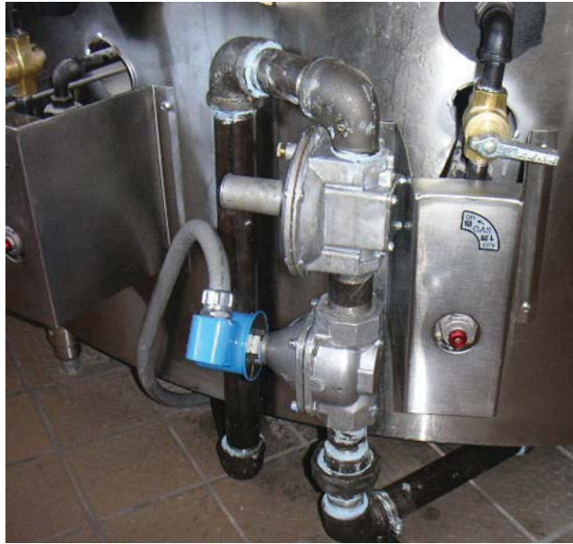
FIGURE 1 A REGULATOR INSTALLED ON THE EXTERIOR OF UNIT
