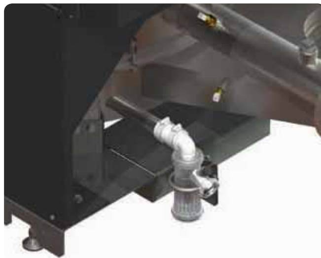
Figure 45 Condensate trap assembly, installed
